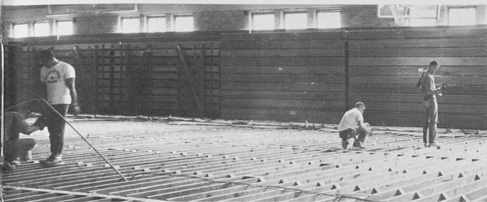
In with the new floor, out with the old as the floor of Gunter gets its first refacing since it was built in 1927.
